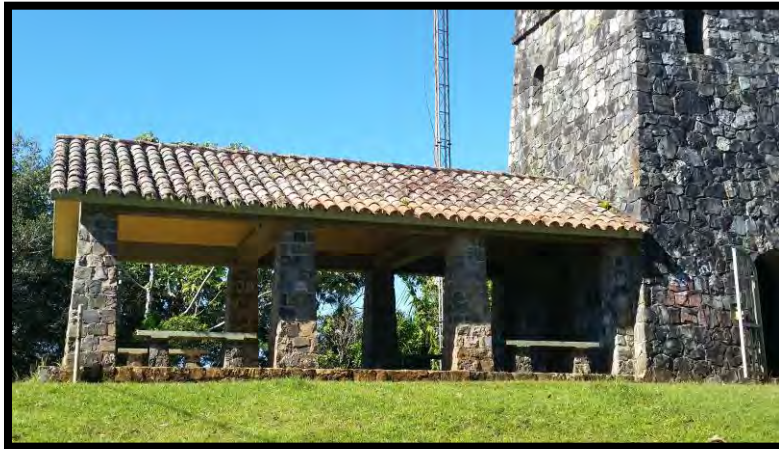
Photo 9. View of the four columns and two of the benches in the eastern picnic shelter taken from the roadway facing southwest.
