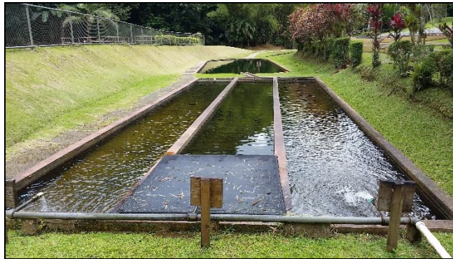
Picture 17. View of the retention tank’s (T26-T28) three pools. Photo taken from the Gazebo area looking east.
